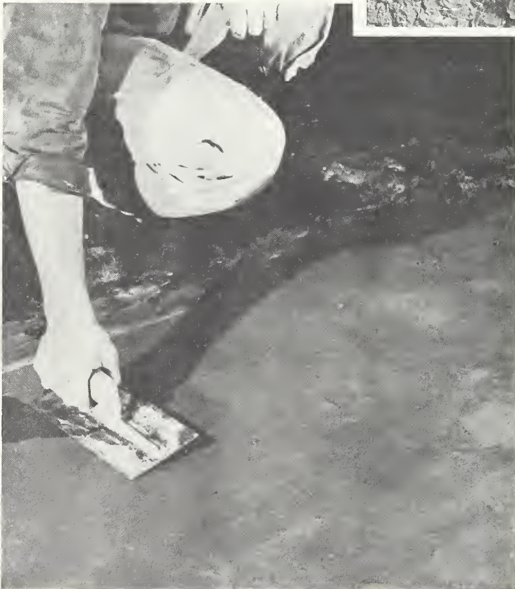
FIGURE 6.5. Trowel finishing latex mortar as a new topping over grout-coated old concrete surface. (Photo courtesy of Paint and Varnish Production.)
