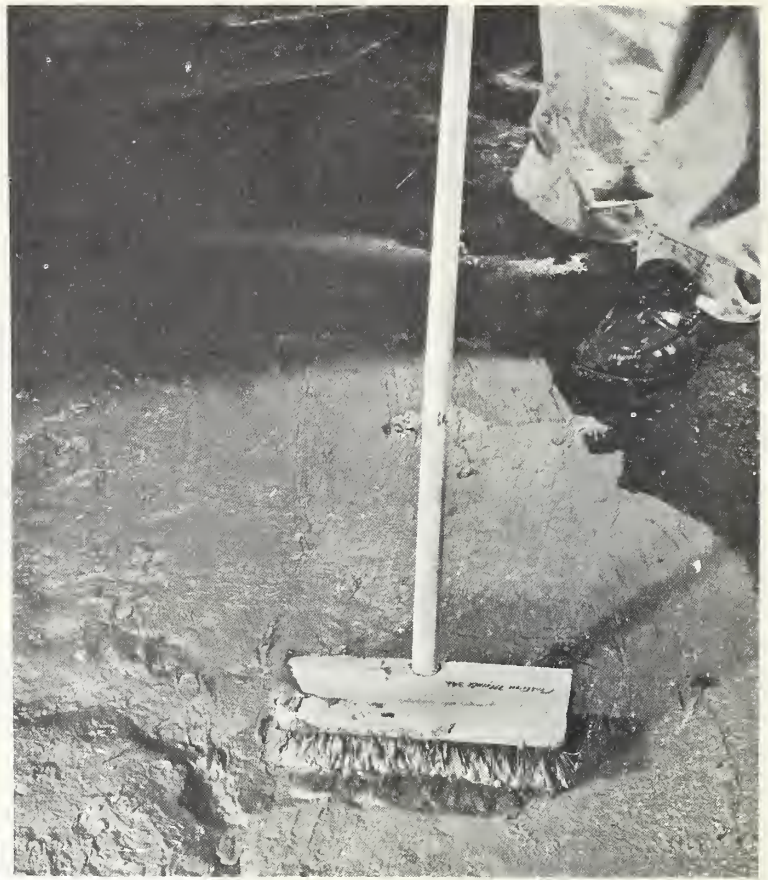
FIGURE 6.4. Spreading a latex grout coat onto a spalled concrete surface. (Photo courtesy of Paint and Varnish Production.)
